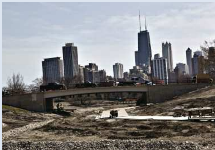
Work to complete the new Nature Boardwalk at Lincoln Park Zoo continues.
